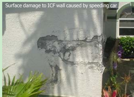
Surface damage to ICF wall caused by speeding car
