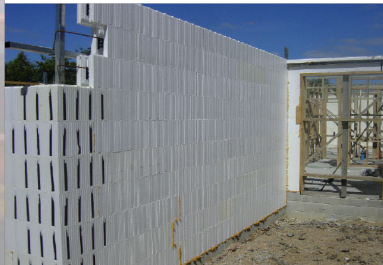
Corner of the house under construction showing the new straight blocks match perfectly with the older corner blocks
